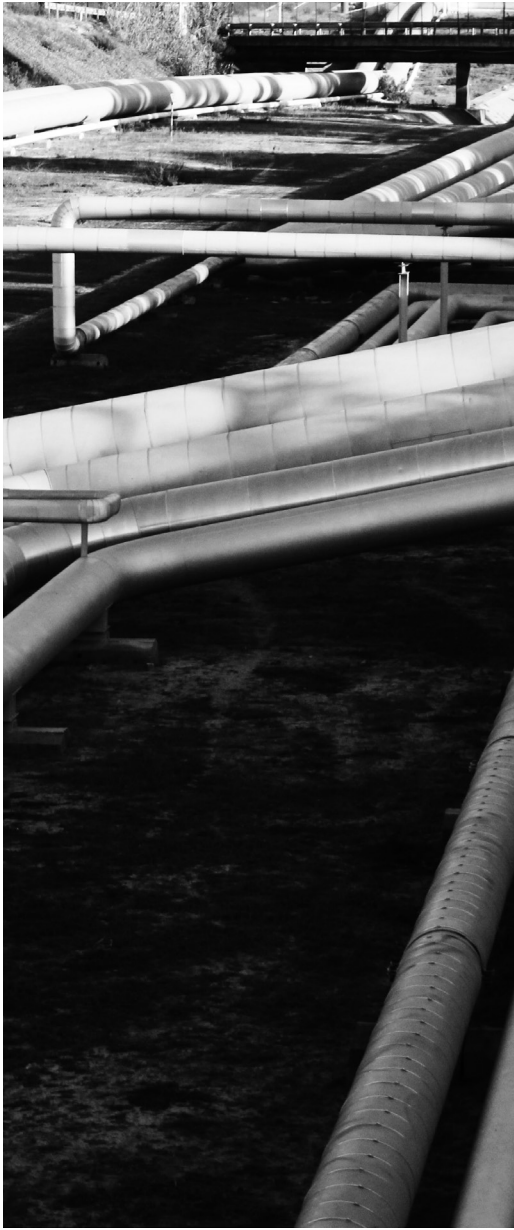
Fig. 3 | Pipelines | Marina Vismara | Sines | 2016
